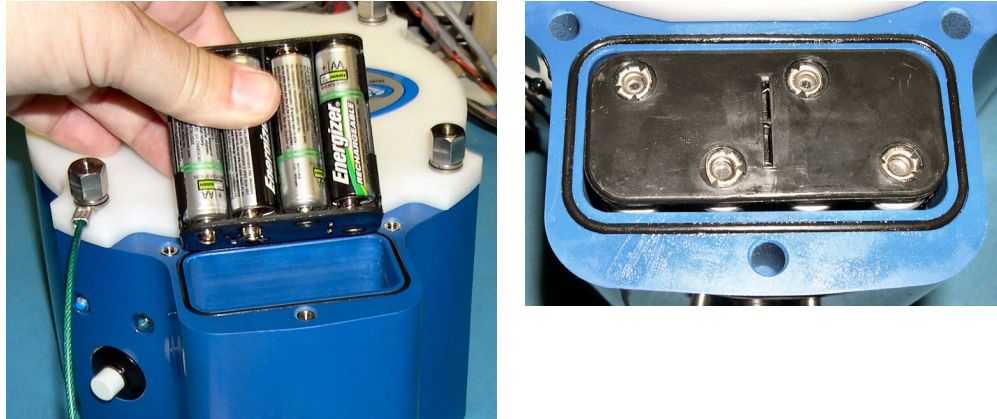
Figure 12. StreamPro Battery Replacement
